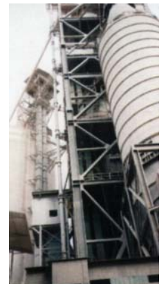
Rexnord® belt elevator feeding raw meal to a pre-heater at a cement plant.
