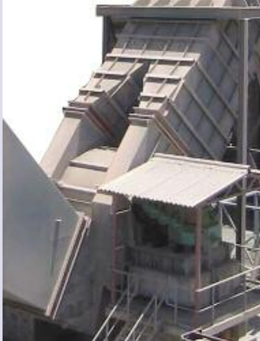
Typical fan arrangement of Fans in Cement Plants.
