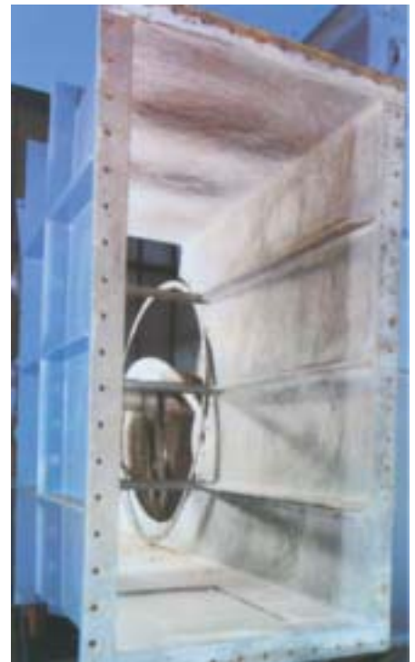
Lead coated inlet box of the scrubber fan.
