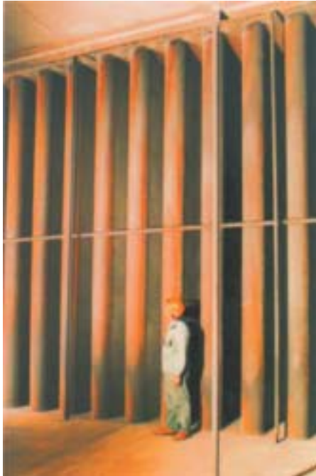
Baffles of the absorptive discharge silencer of a forced draft fan (after approximately 11,000 operating hours); fan performance data are shown on the right. Below:
